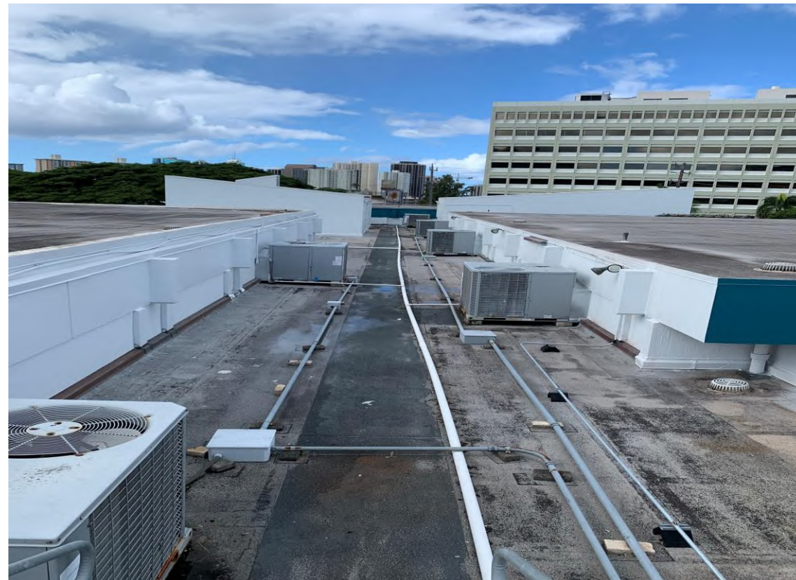
Hawai'i: Roof hardening & wind protection
