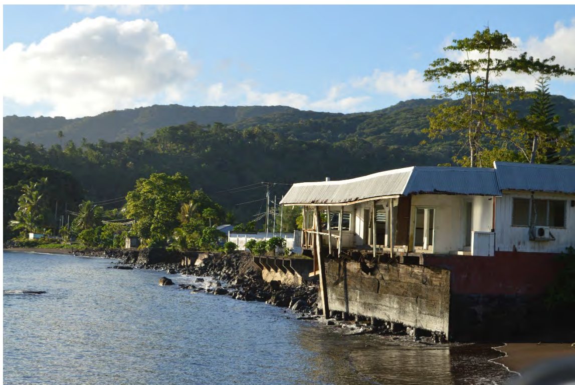
Figure 22: Severely Eroded Shoreline in Village of Leone (Tutuila Island)
