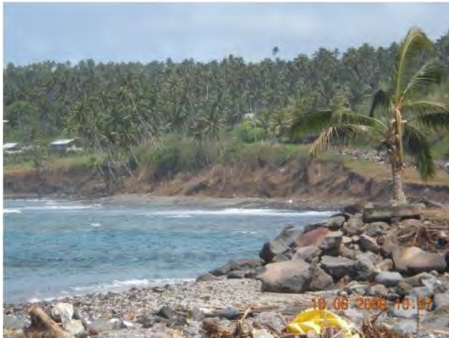
Figure 21: Bluff Erosion in American Samoa
