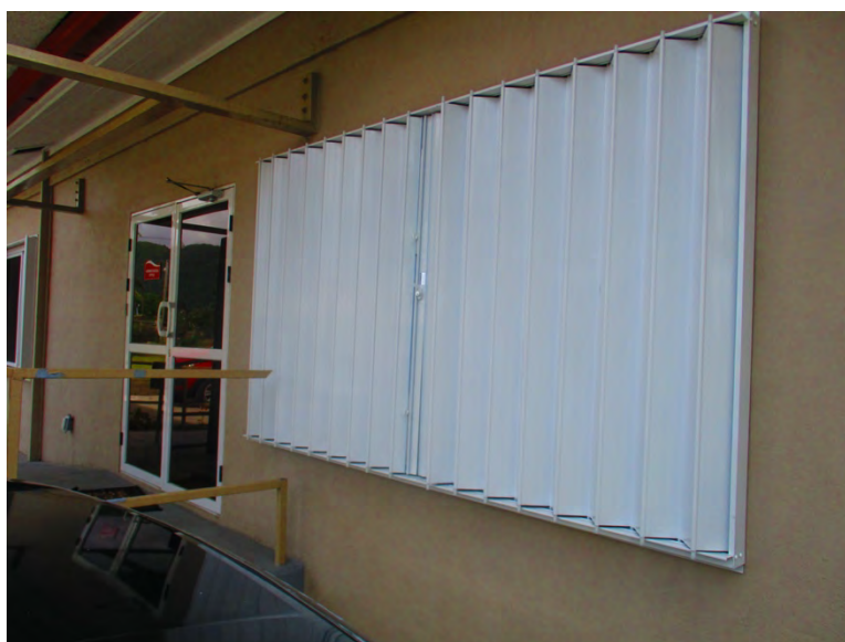
Figure 1 Storm Shutters on the American Red Cross Building, Funding Received Following DR-4192
