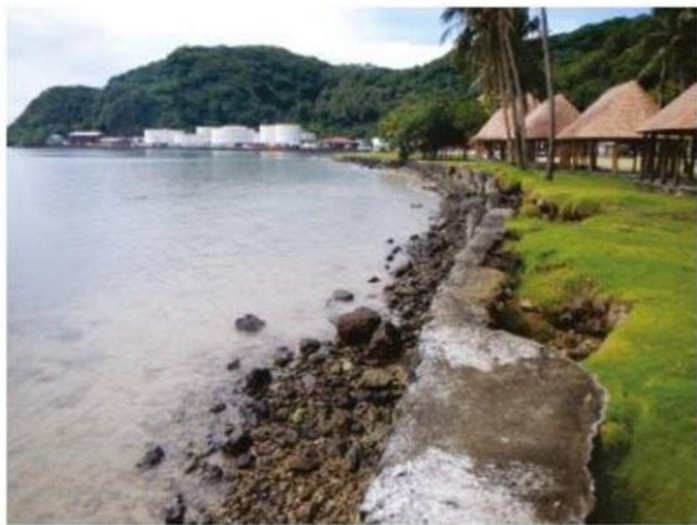
Figure 4. Failing concrete rubble from the American Samoa Shoreline Inventory masonry seawall protecting the park and fales in Reach B2. (USACE 2006, rev.2012).
